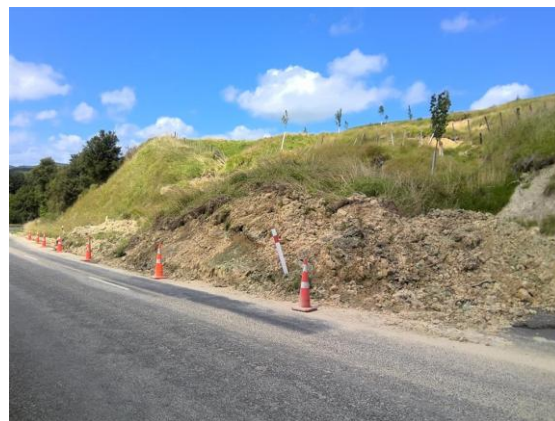
Site on Weber Road where land is moving above the road, drainage and stabilisation planting required
