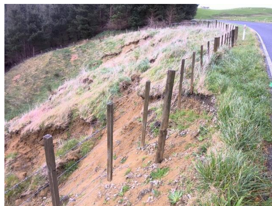
Site on Route 52 where soil is eroding below the road, retaining structure and stabilisation planting required
