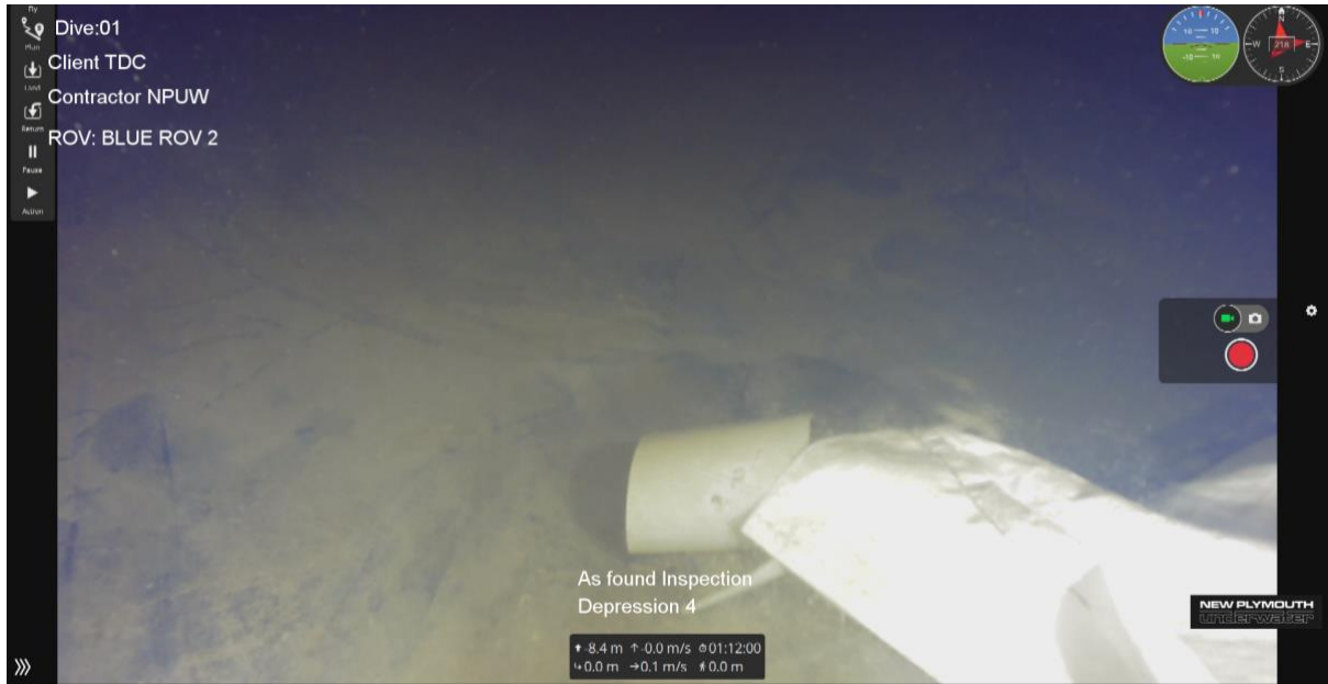
Image 10 Depression 4 Pinhole 5 Butyl tape covering pinhole
